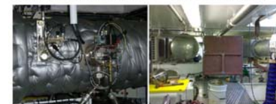
Figure 3.4: Urea injection and PM filter burner.
