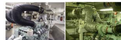
Figure 3.2: Main engine with complete installation.
