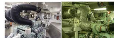
Figure 3.2: Main engine with complete installation.
