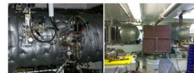
Figure 3.4: Urea injection and PM filter burner.
