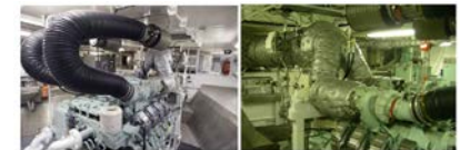
Figure 3.2: Main engine with complete installation.
